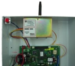
Figure 5. The GSM-200 installed alone in the control panel box
